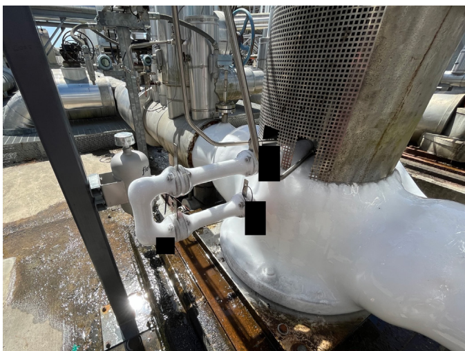
Figure 3. Pump housing with ice accumulation
