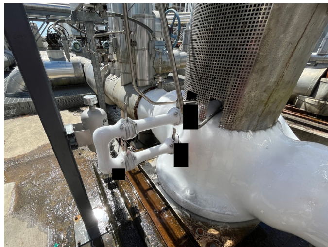
Figure 1. Pump housing with ice accumulation
