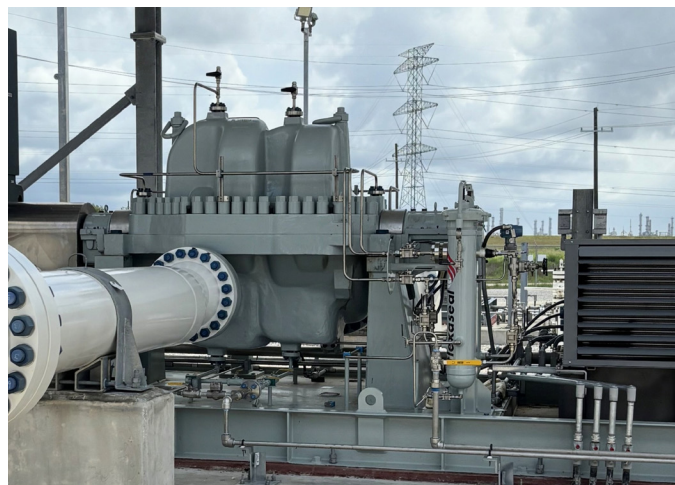
Figure 1. Ethane Mainline Pump
