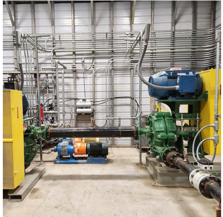
Figure 1. Two RKCS installed in heavy-duty slurry pumps in series.
